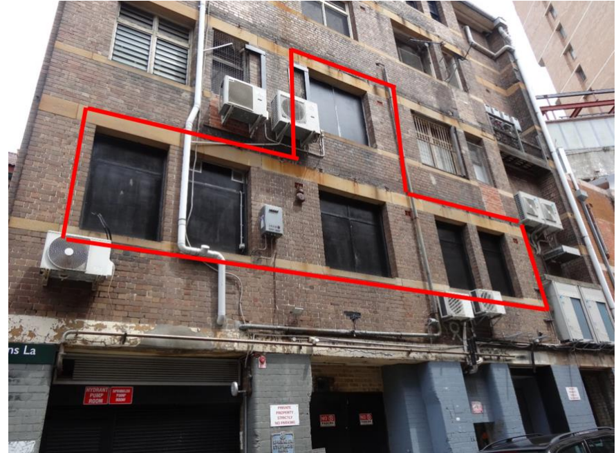
unauthorised works to rear windows
